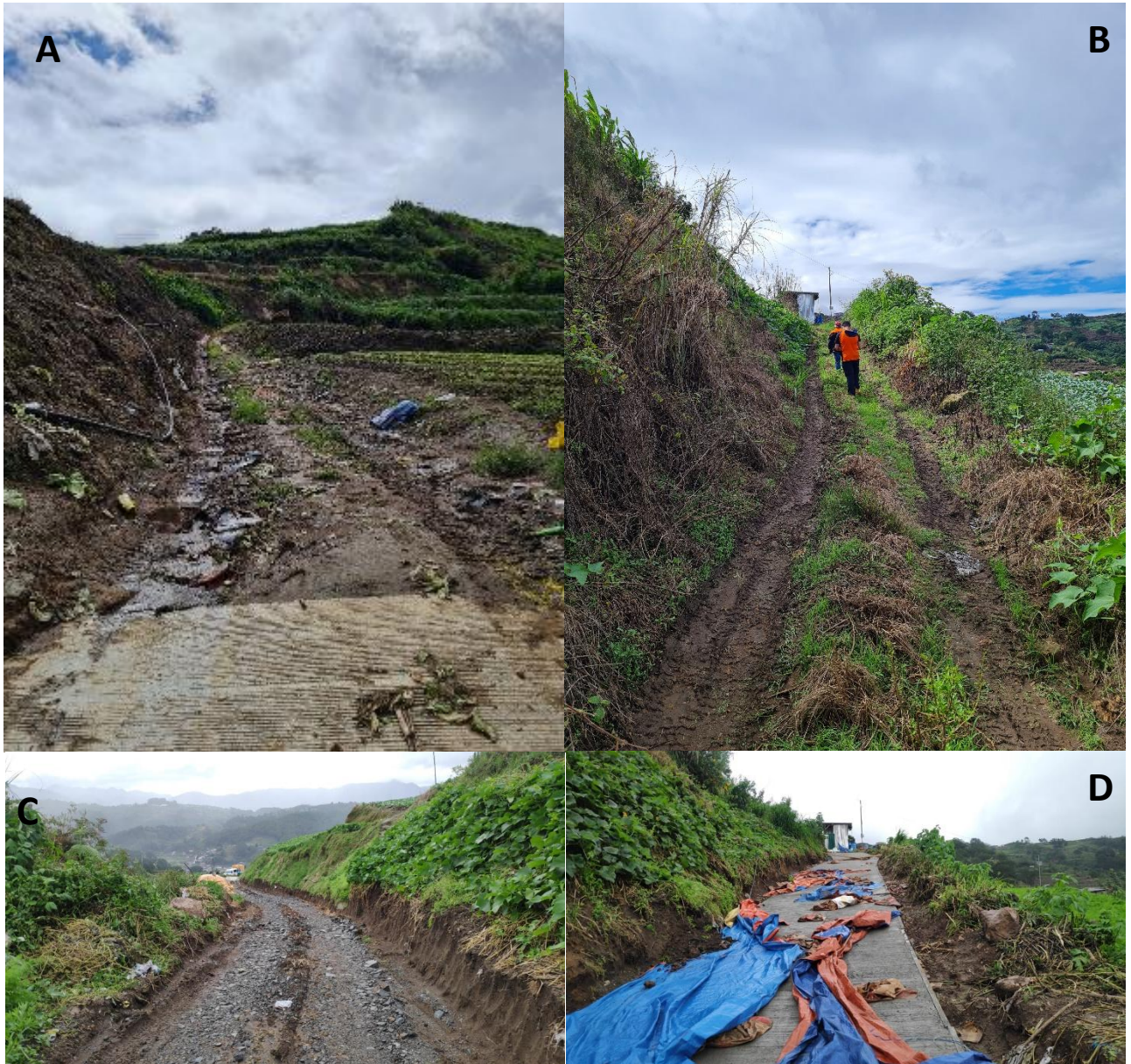
Photo 6. CMDC farm to market road project at Sitio Colocol which will extend the preexisting concrete road to ~100m. Photos A and B show the road condition of the start and end portion of the dirt road to be concreted prior to the construction. Photos C and D show the construction progress of similar areas. Completed concreting of ~20m from the end of the proposed extension (Photo D).
