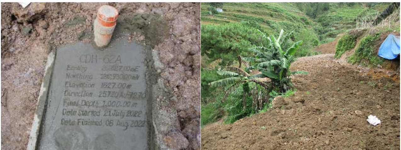
Photo 4. CDH-62A drill site rehabilitation complete. Cemented and plugged collar of CDH-62A (left). Soil backfilled drill pad and access track (right).
