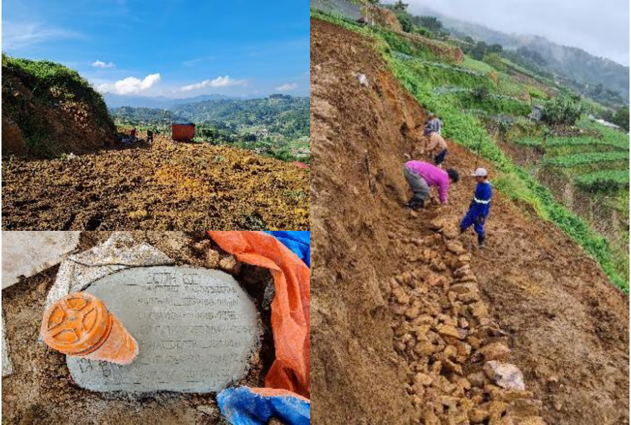
Photo 3. CDH-61 drill site rehabilitation. Riprapping and covering the drill site with soil for farming. PVC pipe inserted in the hole and collar cemented.
