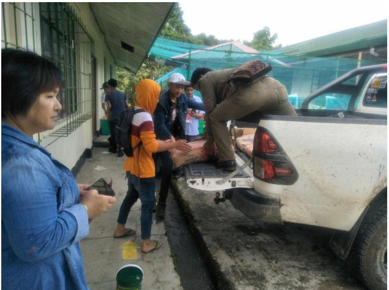
Photo 12. Delivery of 10 bags cement for the construction of washroom at Bedbed National High School.
