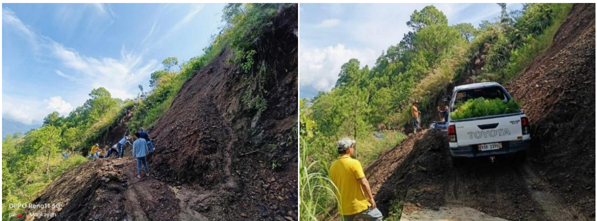
Photo 28. "Bayanihan" clearing operations of a recent landslide along the access road going to the tree planting areas at Brgy. Cabiten.
