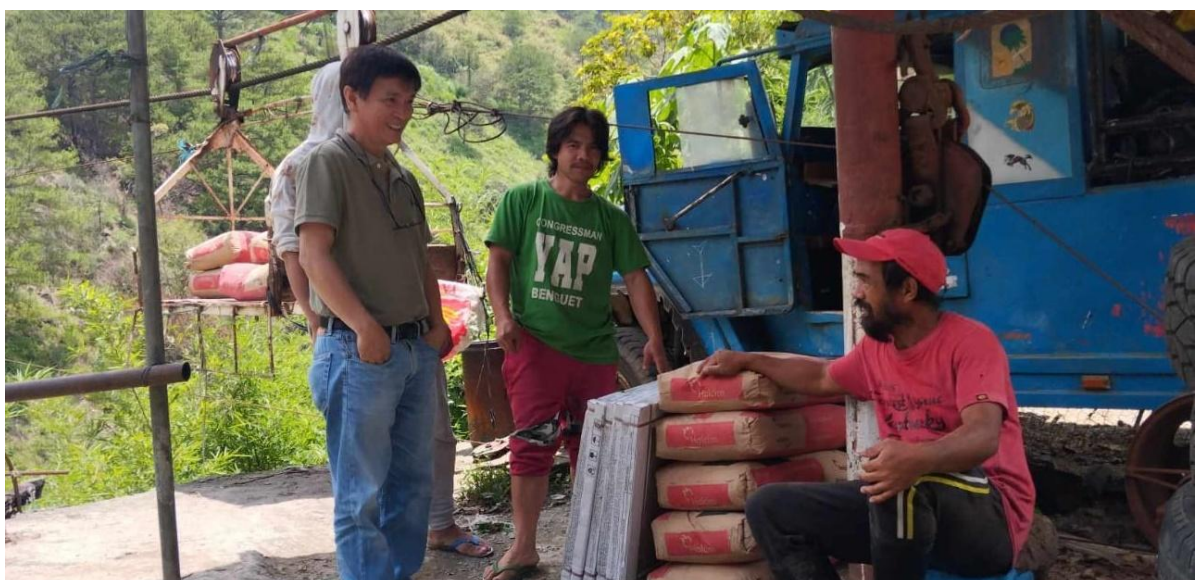
Photo 23. Donated bags of cement and tiles for the repairs of Banooy Taneg – Full Gospel Guiding Light Church received by Pastor Francis Bomowey.
