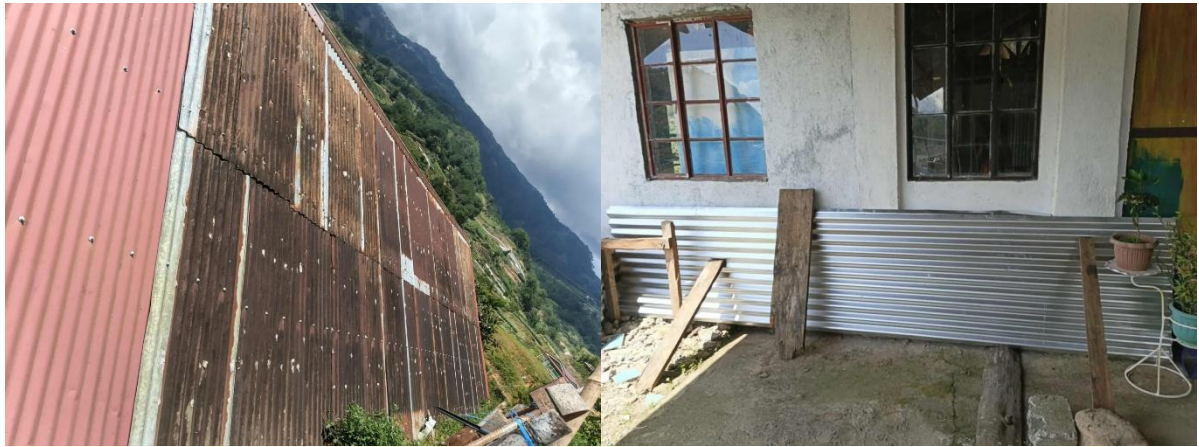
Photo 17. (Left) Current condition of the church’s roof in Sitio Manaba. (Right) Turned over galvanized roofs for the repair of the church.
