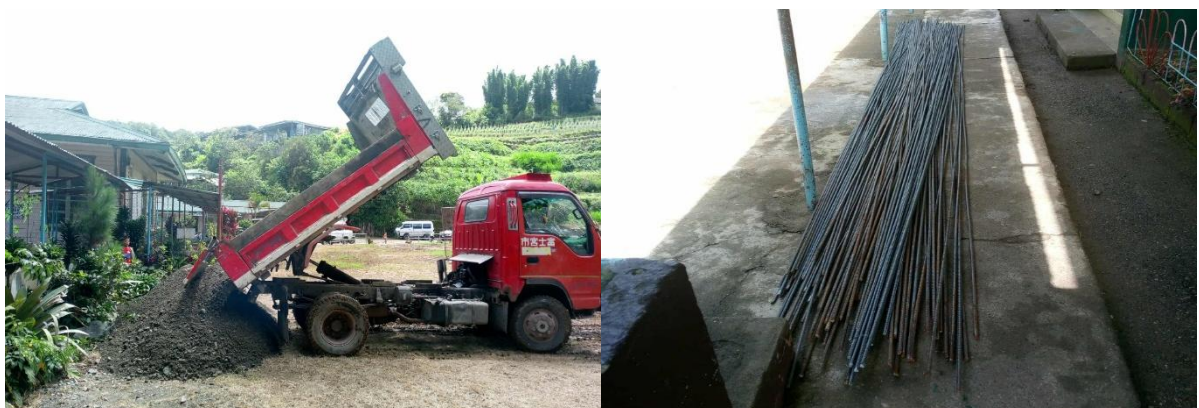
Photo 9. Delivery of sand/gravel and rebars for the rehabilitation of washrooms in Guinaoang Elementary School.
