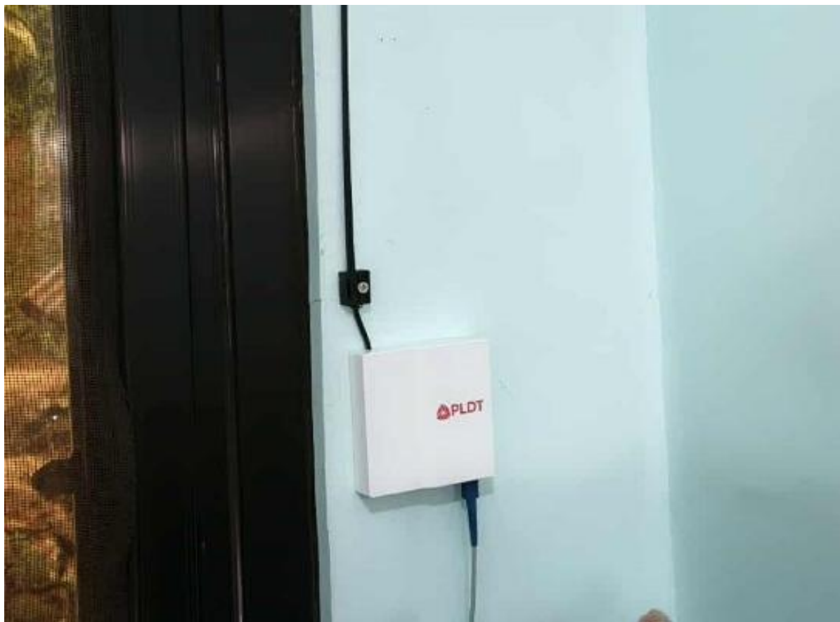
Photo 39. Internet connection installed in Guinaoang Barangay Health Station under the CDP of the company.
